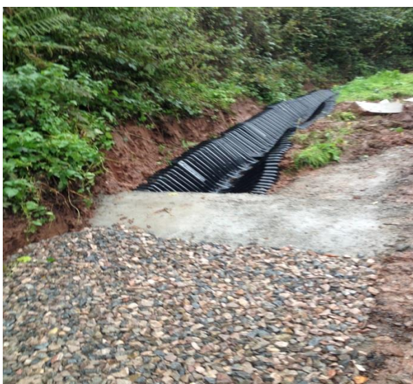
The SmartDitch flows into a culvert at a passing place
