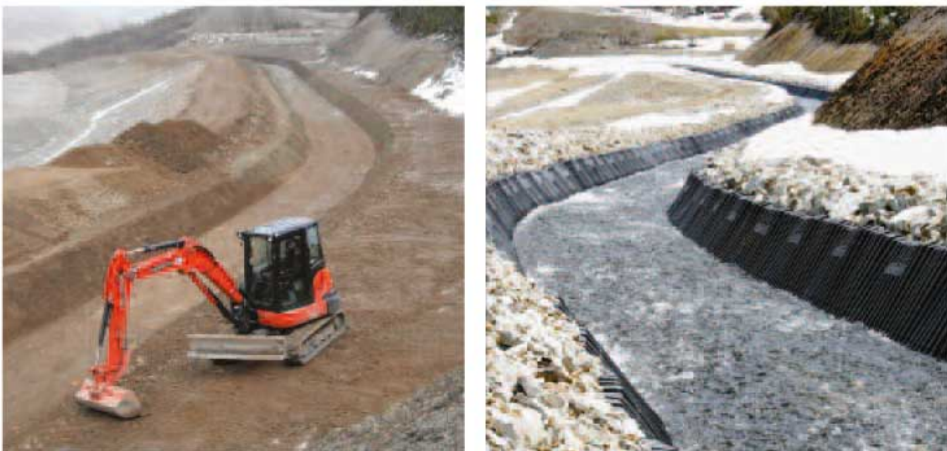
SmartDitch MegaDitch proved to be the only sustainable solution to channel the stormwater/snow melt run off and solve the erosion issues at this mining operation.
